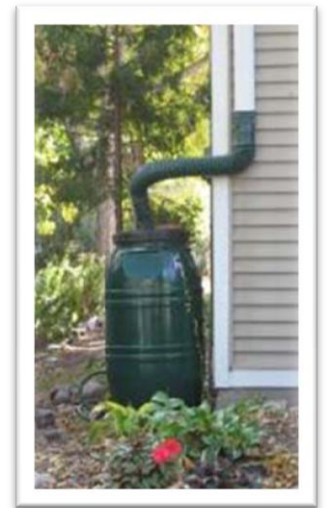
Downspout connection to Rain Barrel
