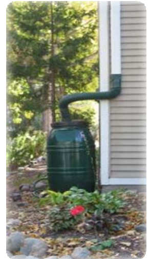
Downspout connection to Rain Barrel
