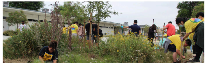
Plymouth School Neighborhood Stormwater Capture Demonstration Project: community drive nature-based project with trees and pervious surfaces for infiltration. Photo by: Amigos De Los Rios.
